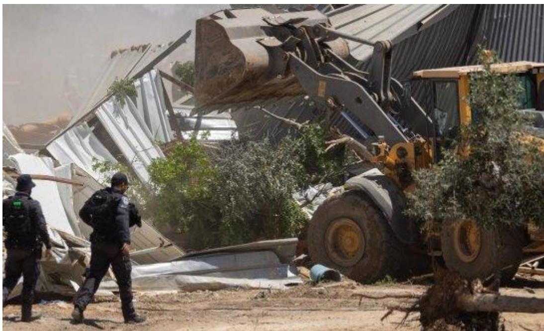
Demolition of Palestinian-Bedouin homes in the Naqab
