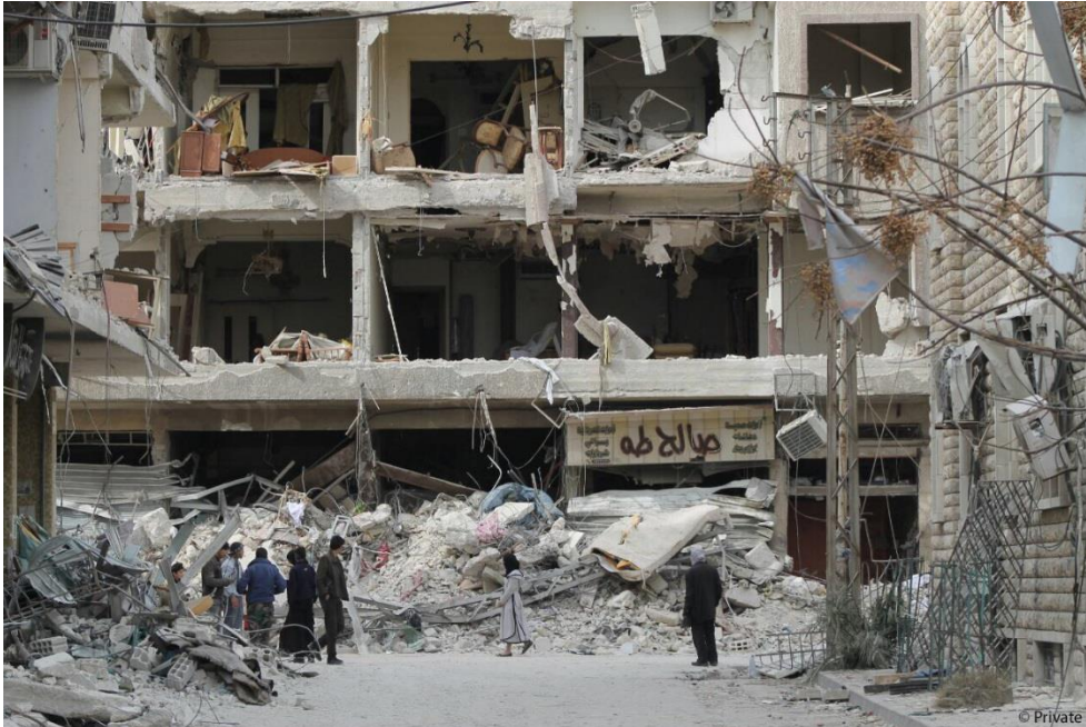
A residential building near the Taha mosque in the Khorshid neighbourhood that was destroyed by a Syrian government air strike on 5 February 2015.
